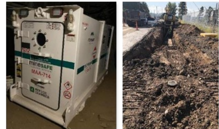
Sanford Underground Research Facility (SURF) Refurbishment and Upgrades HEP Status Fermilab User's Meeting
